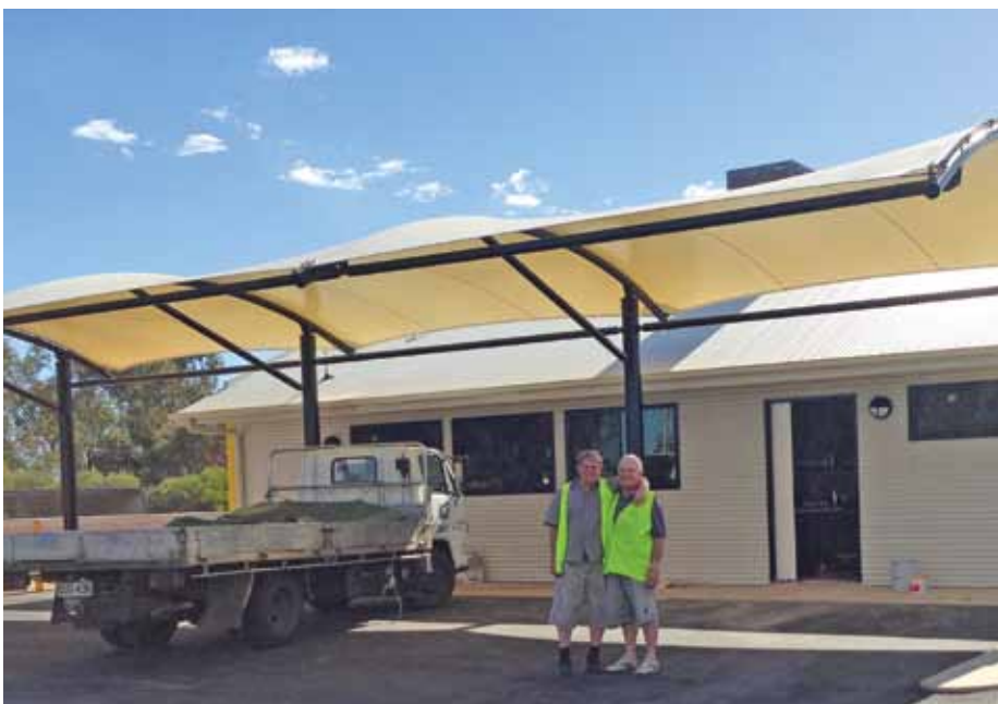
"Acting Site Superintendent" Des Memen and "Temporary Inspector of Works" Frank Petagna take a look at the new awning out front of the new kitchen, which was handy as it was 30 degrees in May!
